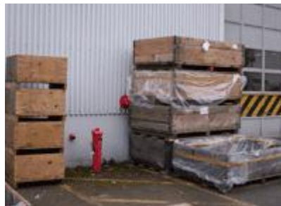
Fire department hose connection is obstructed by pallets
