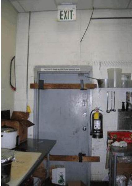
Exit door is blocked and exit sign is not illuminated.
