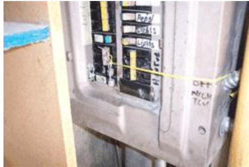
All openings must be covered and breakers that continue to trip should not be tied off.
