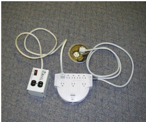
Powerstrips must be plugged directly into an outlet and NOT daisy-chained. This is in violation of the IFC.
