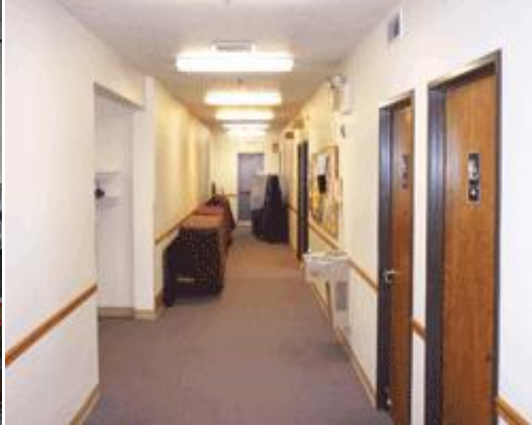
Items are not to be stored in exit corridors
