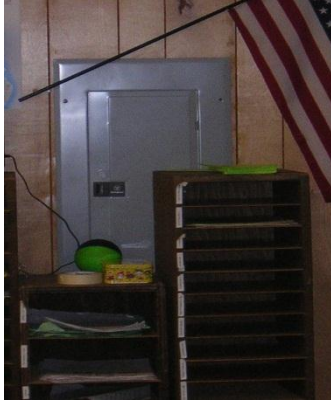
Electrical panel is obstructed.
